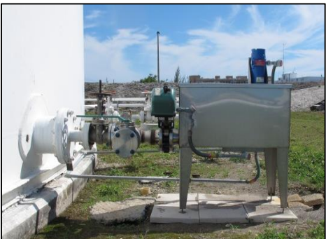
Tanks & Terminals / Dikes & Roof Drains
