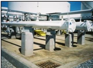
Retention Pads & Drains
