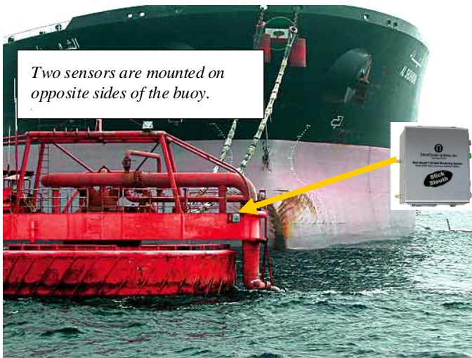
Spill sensors are mounted on the outer circumference of an offshore tanker loading buoy. Two sensors are mounted on opposite sides of the buoy. Oil-on-water alarms are relayed to the tanker vessel to provide near-instantaneous alert of oil spills
