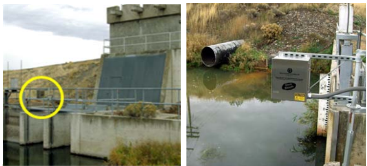
Figure 25. US Army Corps of Engineers utilizes a network of sensors at critical pump stations (lift stations) to prevent potential oil spills in city drainages from getting into a major river where Salmon spawning occurs. Alarm signal automatically disables the pumps and remote alarm is received at the local 24-hour manned control center. 5-unit system has been in operation for several years.
