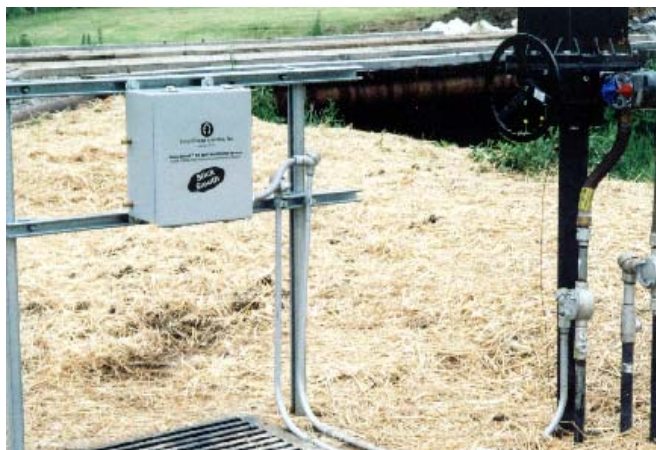
Figure 4. Oil detector monitoring for compressor oil in a storm water sump at a natural gas pipeline compressor station. Real time alarm is sent to company headquarters and valve closes automatically upon detection of oil.
