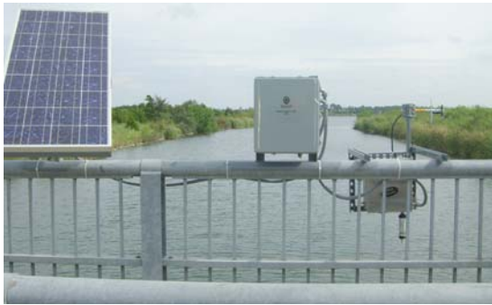
Figure 12. Real-time monitoring at industrial outflow point, where discharge enters a river and then a municipal lake. Utilizes solar power and wireless (RF) alarm/data transmission for instantaneous alert to facility control room.
