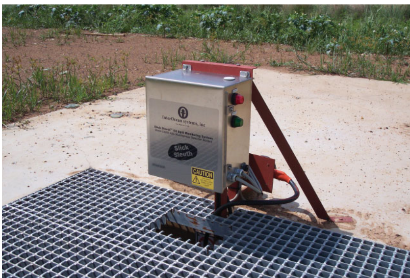
InterOceans Systems oil-spill detection monitor
